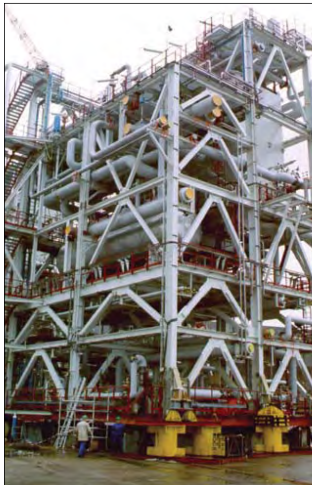
The Karsto gas treatment facility in Norway is another example of KBR's ability to design and construct major processing plants on schedule and with an exemplary health, safety, and environmental record.
