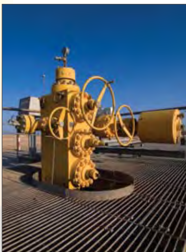
On-stream since July 2004 with the help of KBR and its joint venture partners, In Salah Gas project produces around nine billion cubic meters of gas per year.
