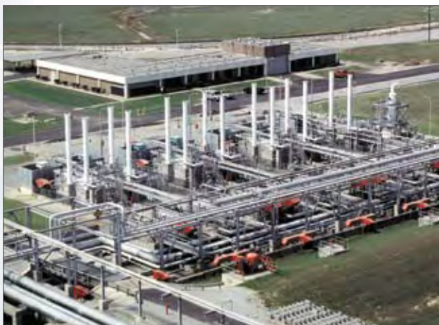
Trunkline LNG Company in Lake Charles turned to KBR when they needed design and EPC for their terminal constructed 25 miles inland from the Gulf of Mexico on an industrial canal.
