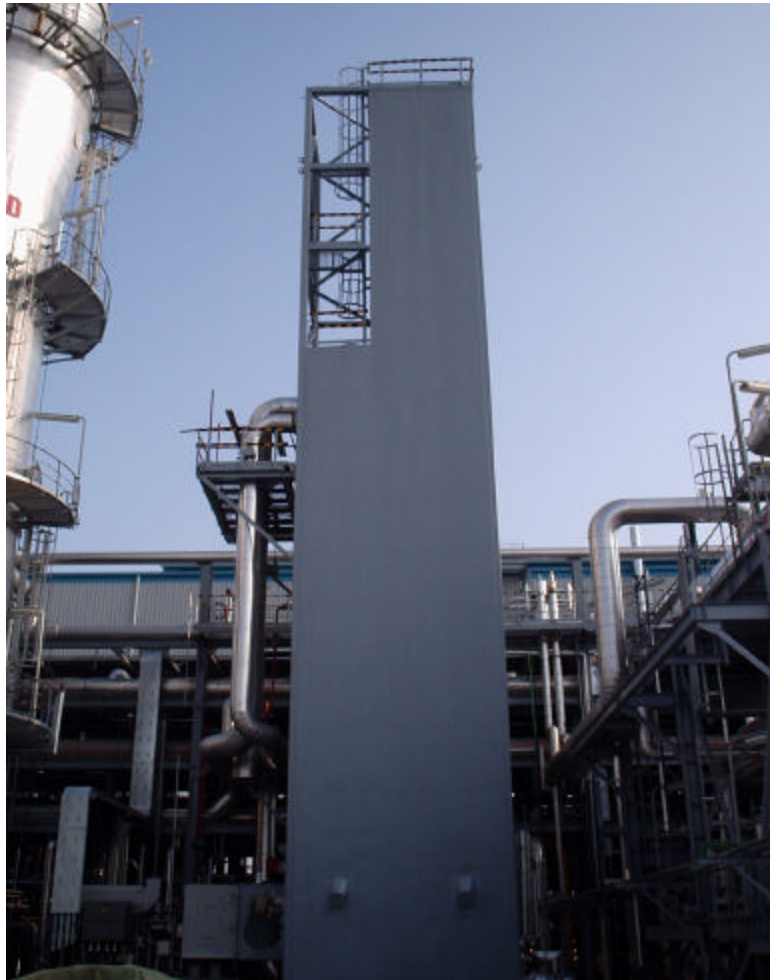
PHOTO 3: KBR PURIFIER COLD BOX AT A RECENTLY BUILT PLANT
