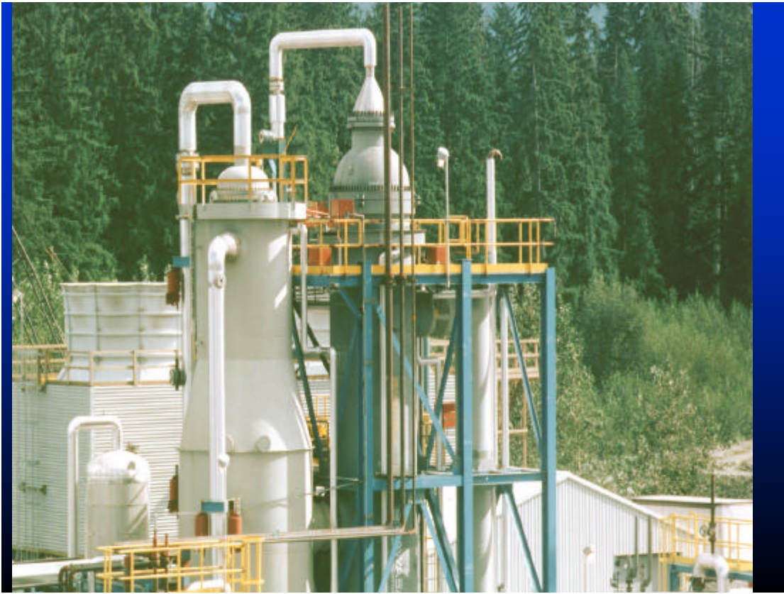
PHOTO 1: KRES™ AT PLANT IN CANADA, WITH AUTOTHERMAL REFORMER ON THE LEFT AND REFORMING EXCHANGER ON THE RIGHT.
