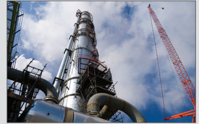
SASOL's olefins plant in Secunda, South Africa is the first commercial application of SUPERFLEX technology. The plant achieved a successful start-up in 2006.
