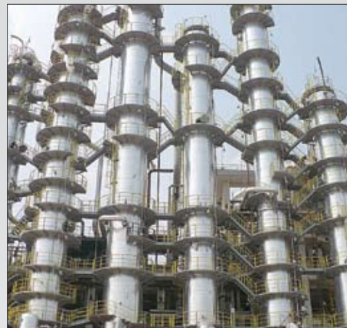
KBR's phenol technology team provides services to clients including technology licensing and support in the initial planning phase of projects, through process design, engineering and construction of phenol plants.
