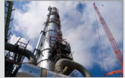
SASOL's olefins plant in Secunda, South Africa is the first commercial application of SUPERFLEX technology. The plant achieved a successful start-up in 2006.
