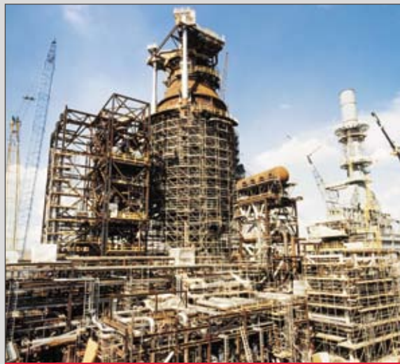
EPC, start-up support and managed all subcontracts for Syncrude Canada Limited's grassroots Vacuum Distillate Unit, plus debottlenecking of six operating units in the Upgrader.
