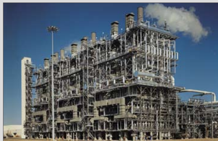
Construction of Dow Chemical's Canada Inc.'s grassroots 1.2 billion pounds per year ethylene plant complete with fractionation facilities, including six ethylene cracking furnaces.
