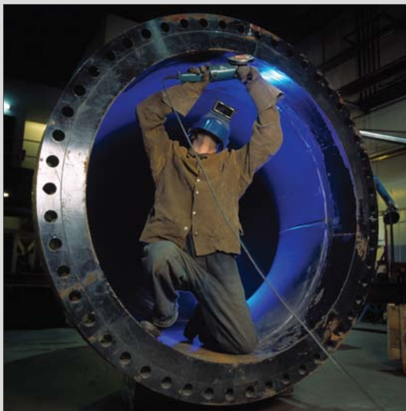
KBR has a history of adapting to the client challenges and project needs. Upon expansion in 2008, our five-bay, 600,000 WDI per year pipe fabrication shop in Edmonton will increase capacity by 50 percent.
