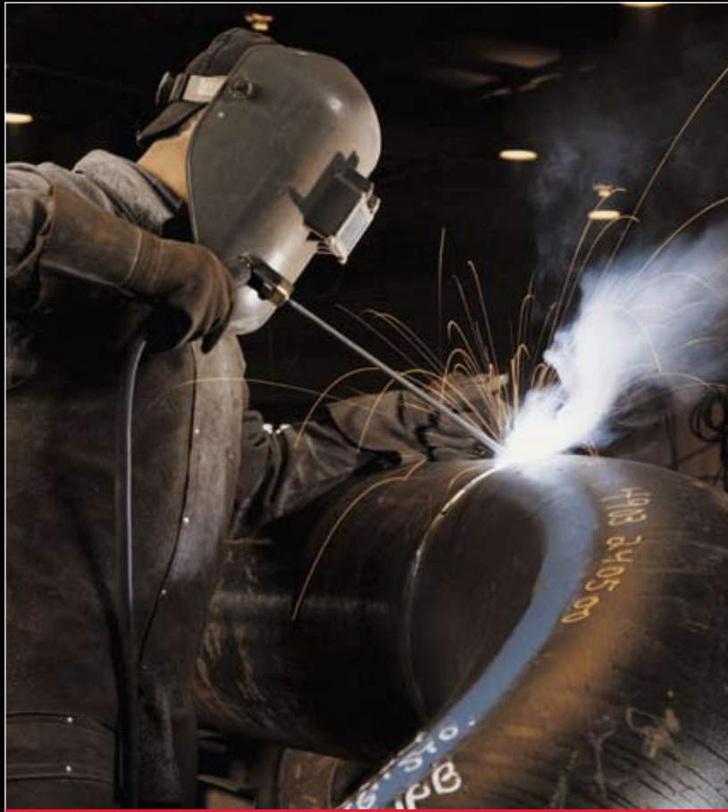
KBR's highly trained specialists adhere to HSE standards in all on-site construction, turnarounds and modular assembly and pipe fabrication projects.
