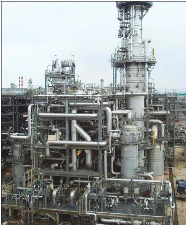
Nigeria LNG - KBR, along with its joint-venture partners, has helped Nigeria LNG achieve an unprecedented rate of growth through four successive engineering, procurement, construction, and commissioning projects, creating one of the world's largest LNG facilities.
